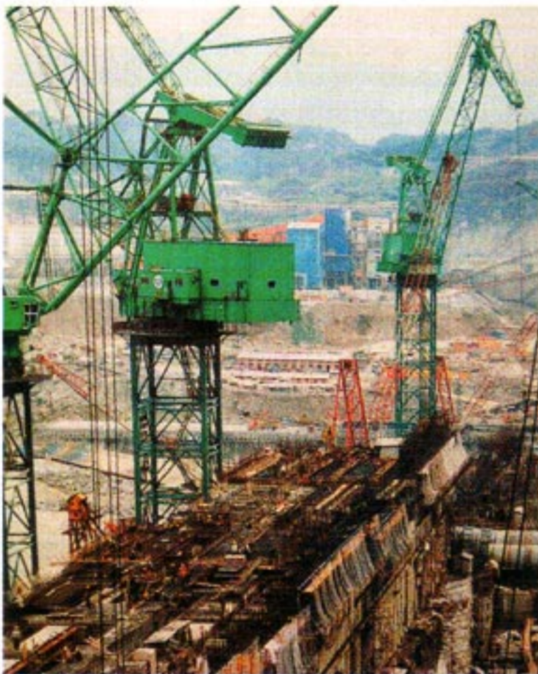
Five MQ2000 cranes with double lever booms were engaged at the massive Three Gorges project with up to 100m hook height on rail travelling portal and 71m maximum working radius
